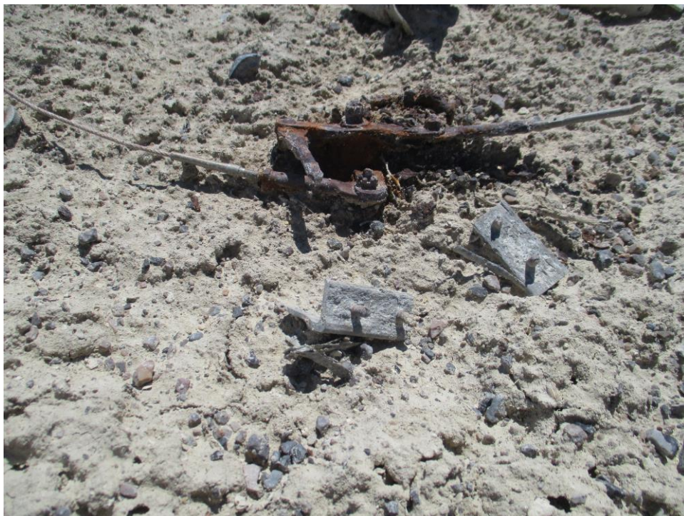
These control cables were also damaged by fire
