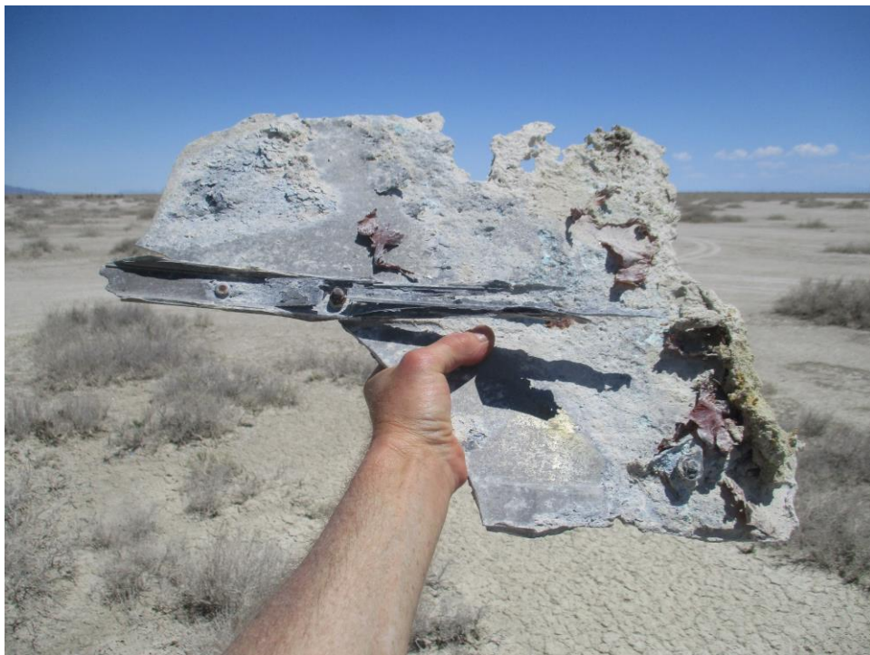
Fire damage is evident on this aluminum panel
